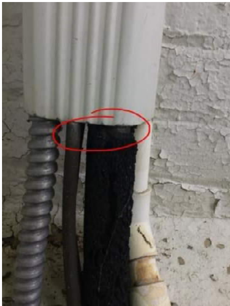
Refrigerant line set rubbing
