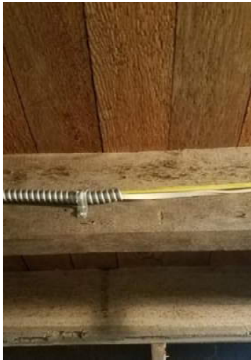
Example of inappropriate wiring found in basement
