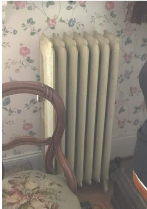
Cast Iron Radiator
