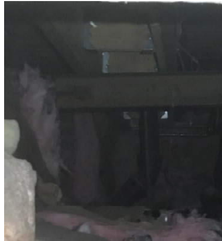
Example of Cast Piping
