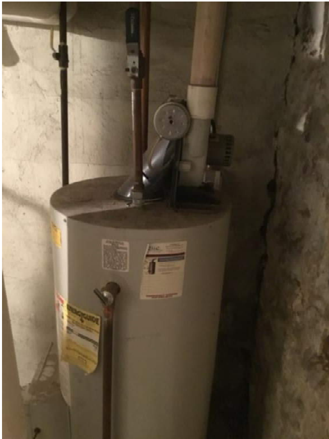
Gas fired water heater
