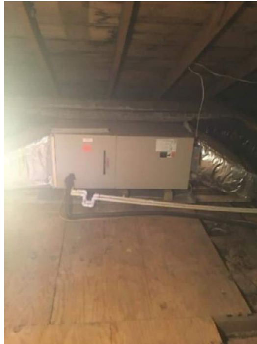
AC evaporator and fan in attic
