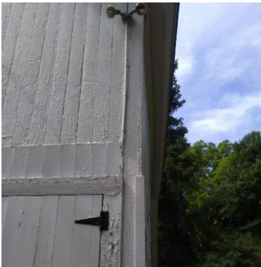
Picture of carriage house paint siding showing wear
