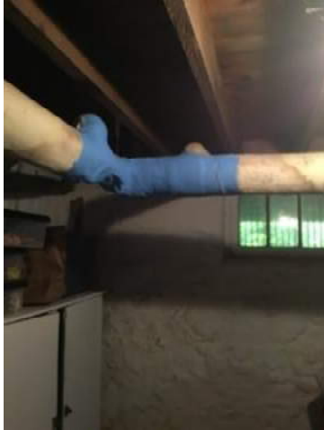
Steam piping - example of possible asbestos insulation
