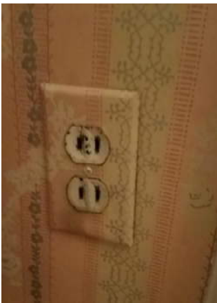
ungrounded receptacle – second floor bedroom
