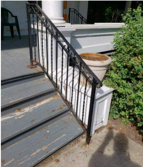
Rusted railing, wood sections rotted/failing, repair/paint.
