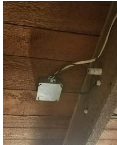
Example of inappropriate wiring found in basement
