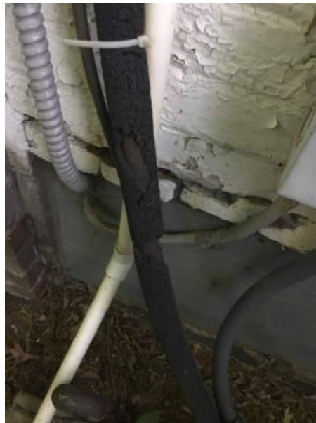
Degraded Refrigerant Line set Insulation
